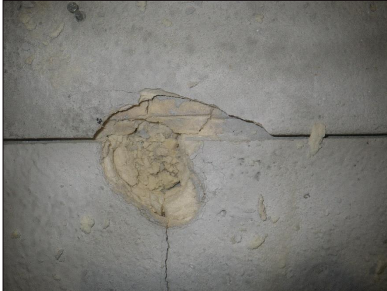
Photo No. 5 2nd Location – Top of Tile at 22 Impacts
