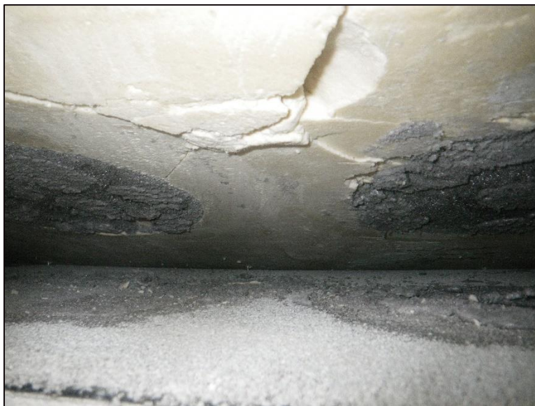
Photo No. 2 1st Location – Underside of Tile at 31 Impacts
