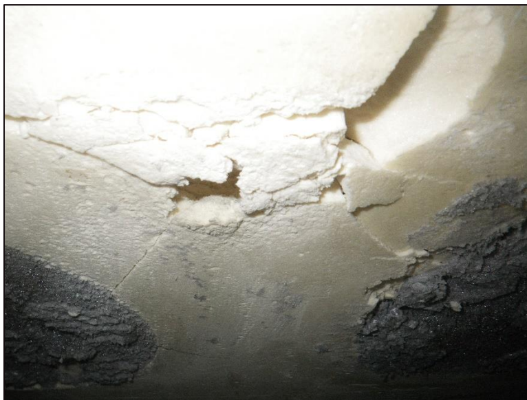
Photo No. 4 1st Location – Underside of Tile at 51 Impacts
