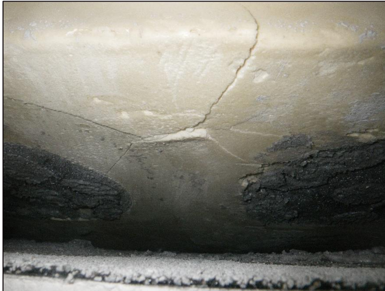
Photo No. 1 1st Location – Underside of Tile at 20 Impacts
