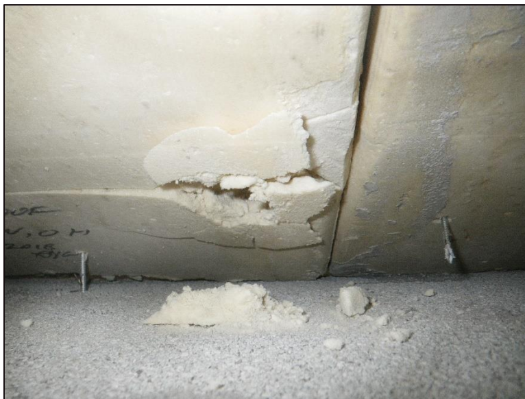
Photo No. 6 2nd Location – Underside of Tile at 22 Impacts
